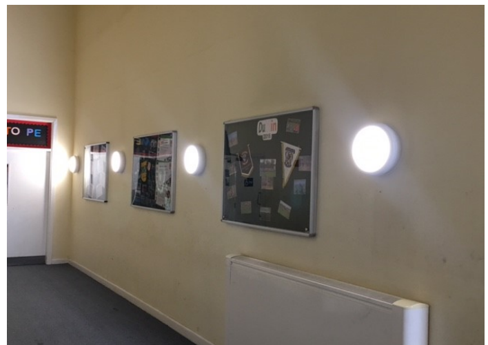
The Picture above shows the Sports Centre corridor fitted with 28w LED Bulkheads
